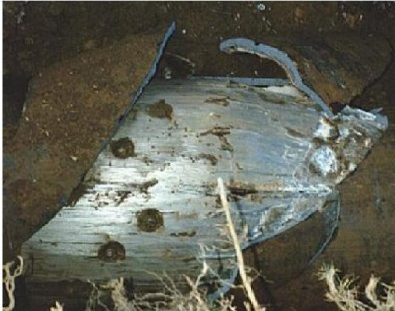
PE pipe bursting head breaking open cast iron pipe at an excavation – Photo courtesy of CLM Trenchless.
