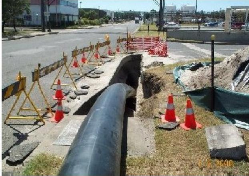
Slip Lining with DN500 PE, Botany NSW (photo courtesy of CLM Trenchless)
