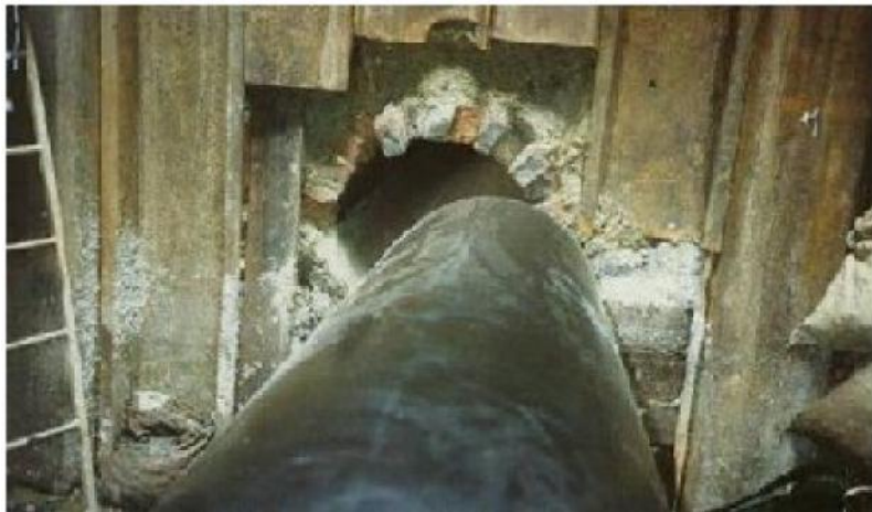
PE liner about to enter an old brick sewer (photo courtesy of Vinidex)
