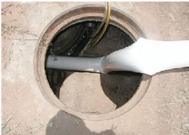
“Ex” Pipe PVC liner system entering a sewer access chamber – Courtesy of Vinidex.
