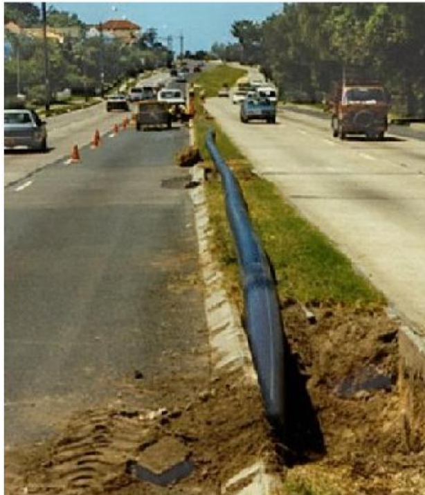
PE being drawn behind pipe burster on Pittwater Rd, Sydney - Photo courtesy of CLM Trenchless.
